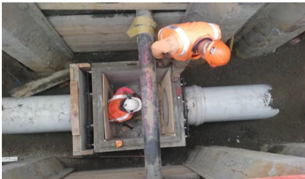
The wastewater manhole being constructed at the intersection of Darvel Street and Riccarton Road.
